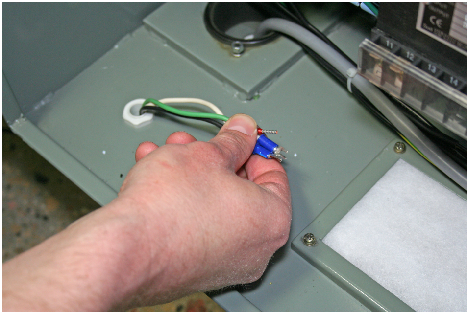
Figure 8: Automatic oiler wires routed through the cord grip in the electrical cabinet.
