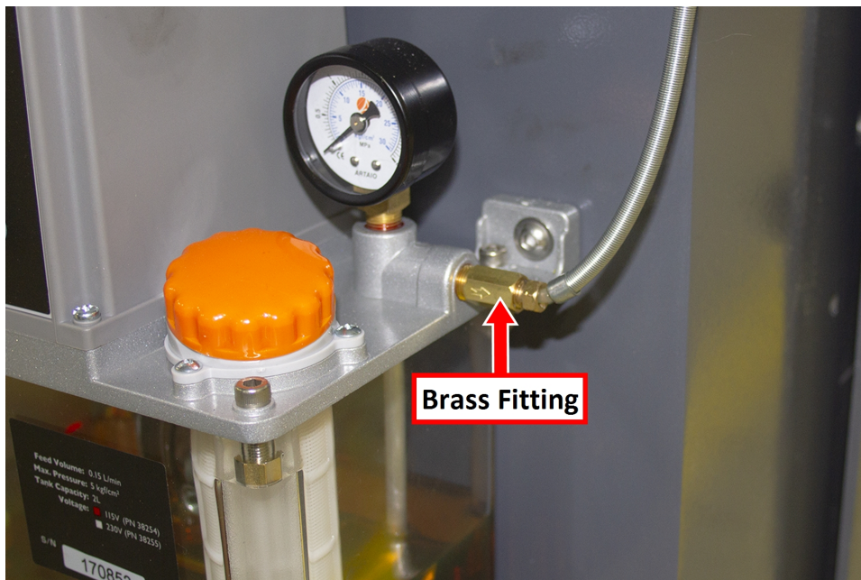
Figure 2: Brass fitting on the automatic oiler.
