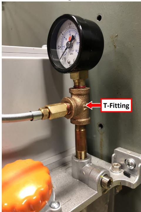
Figure 3: T-fitting installed on the automatic oiler.
