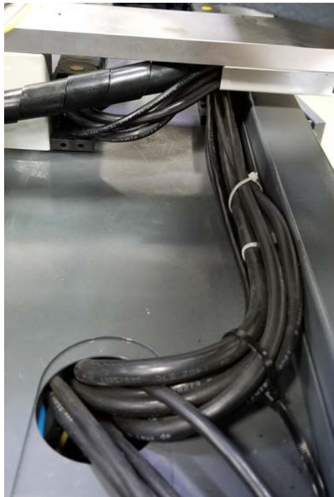
Figure 5: Cable routing through the hole on the top of the electrical cabinet.
