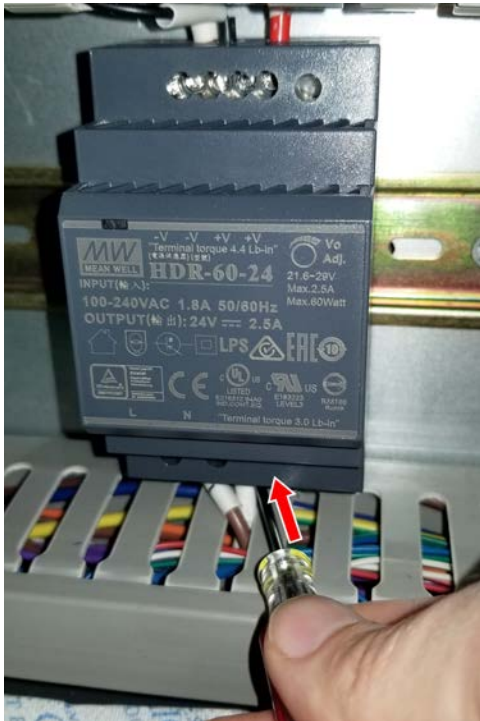
Figure 2: Existing power supply attached to the DIN rail.
