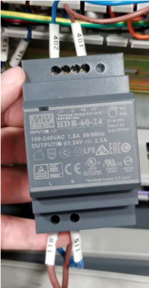
Figure 5: Wire connections made on the replacement power supply.
