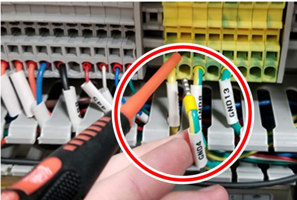
Figure 4: Ground wire in the electrical cabinet.
