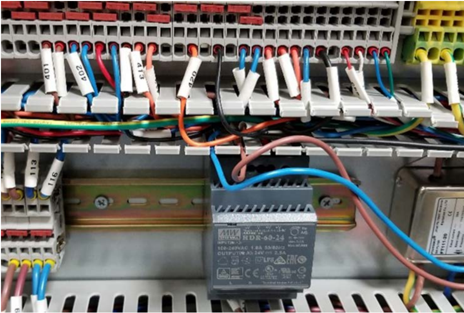
Figure 6: Replacement power supply mounted on the DIN rail.
