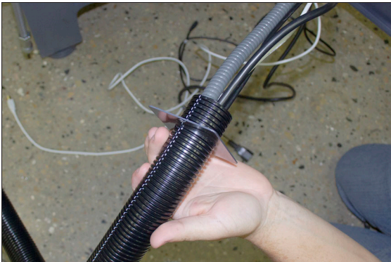
Figure 4-194: Loose end of corrugated tubing and all cords put through the access panel.
