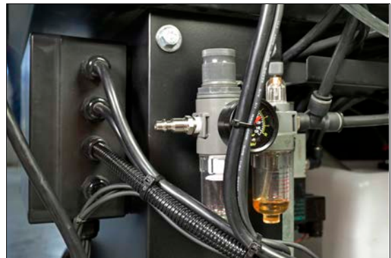
Figure 4-18: Provided air fitting installed on the FRL.
